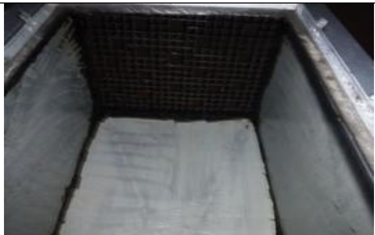
7. Duct abvoce the fan after
