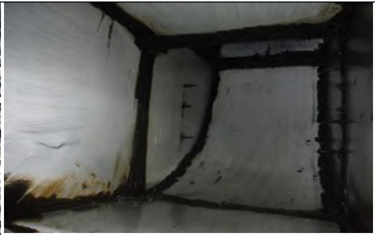
7. Duct abvoce the fan after
