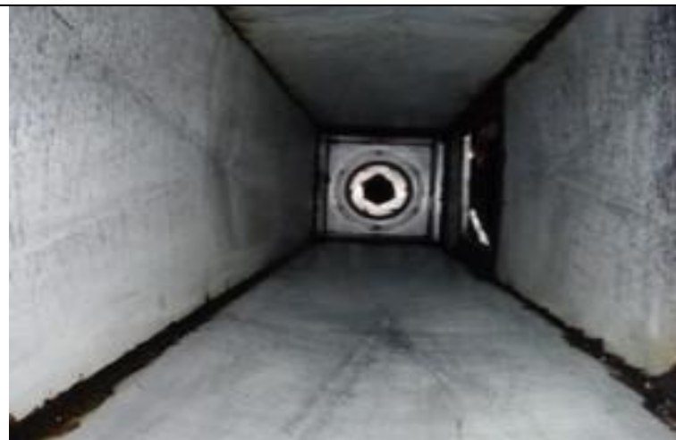
5. Ductwork Upstream of Fan after
