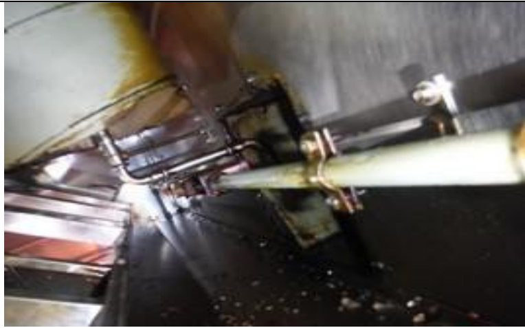
1 Canopy plenum (2 nd Extract)before
