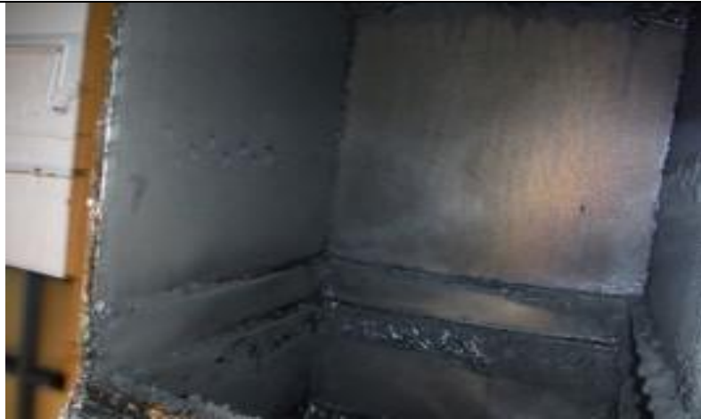
4. Ductwork Midway between canopy and fan before
