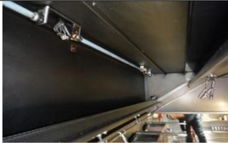
1 Canopy plenum (Main Extract) after
