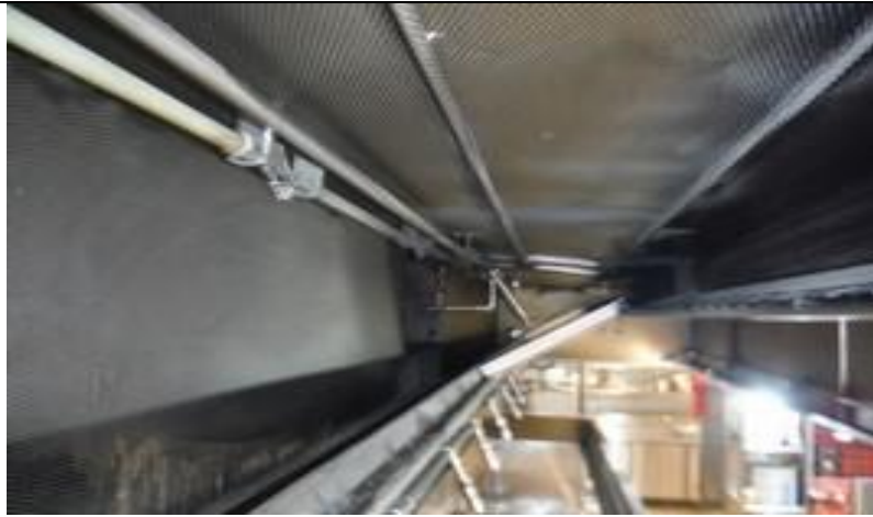
1 Canopy plenum (Main Extract)before
