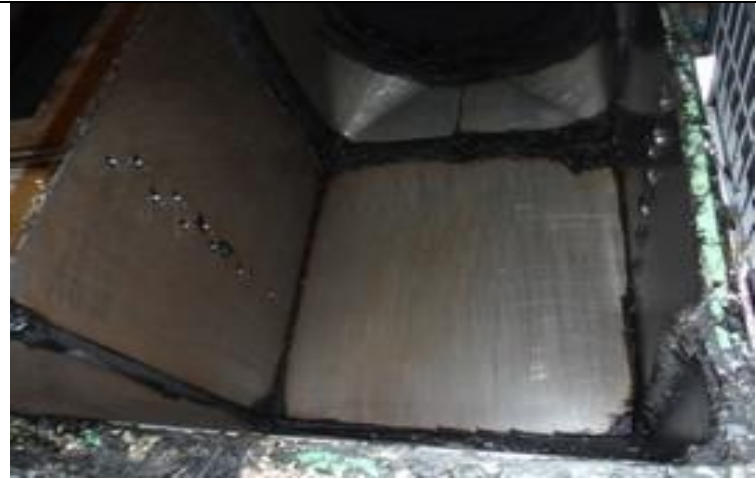
4.Ductwork Midway between canopy and fan after
