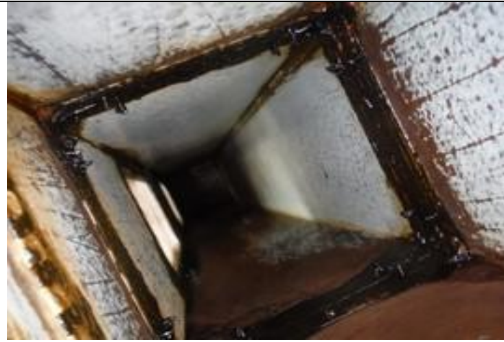
4. Ductwork Midway Between Canopy and Fan After
