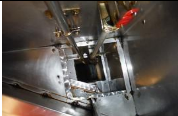
1. Canopy plenum (Basement Extract) Afer
