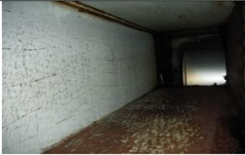
4. Ductwork Midway Between Canopy and Fan Before
