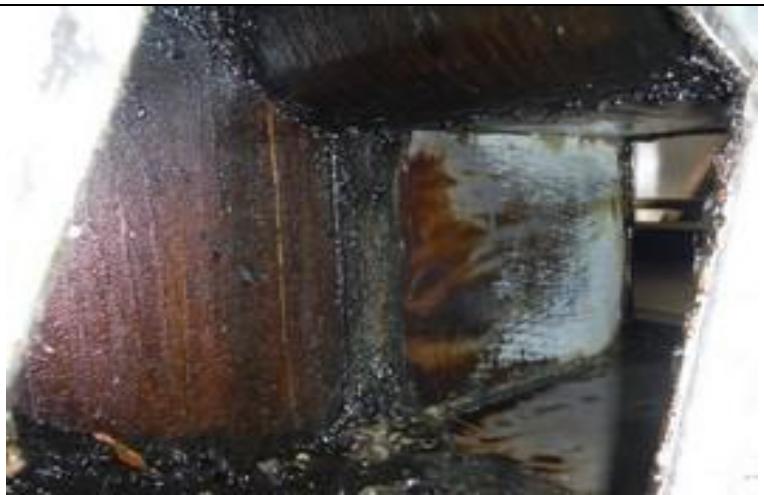
4 Ductwork Midway between canopy and fan before
