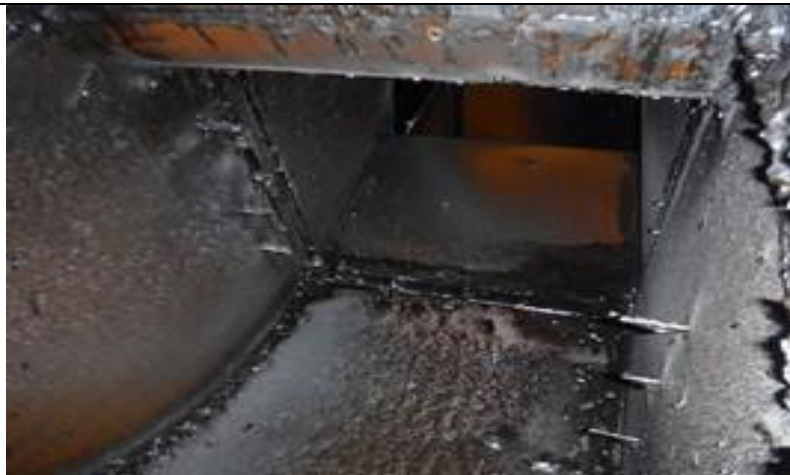
7. Duct above the fan before
