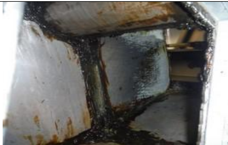
4 Ductwork Midway between canopy and fan after
