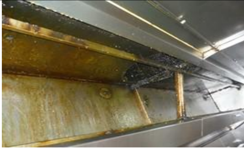
1 Canopy plenum (Main Extract)before
