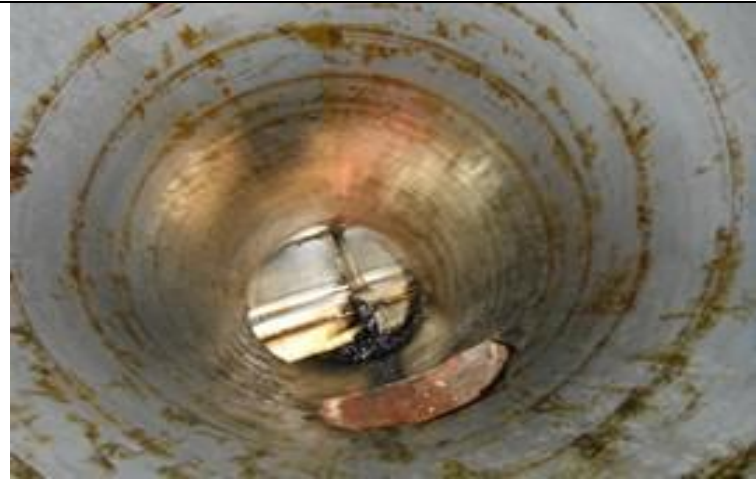
3.Ductwork 3M/midway from canopy after
