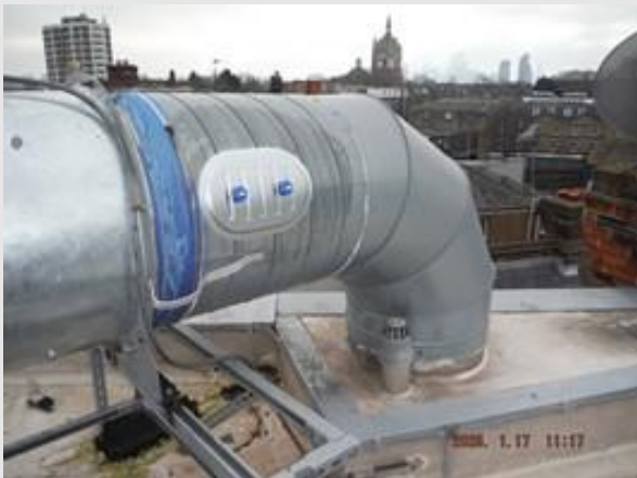
PICTURE SHOWS DUCT DROPS DOWN INTO THE RISER SHAFT - FUTURE INSPECTION REQUIRED WITH MANAGEMENT OF THE BUILDING TO CHECK IF RISER IS ACCESSIBLE FOR CLEANING
