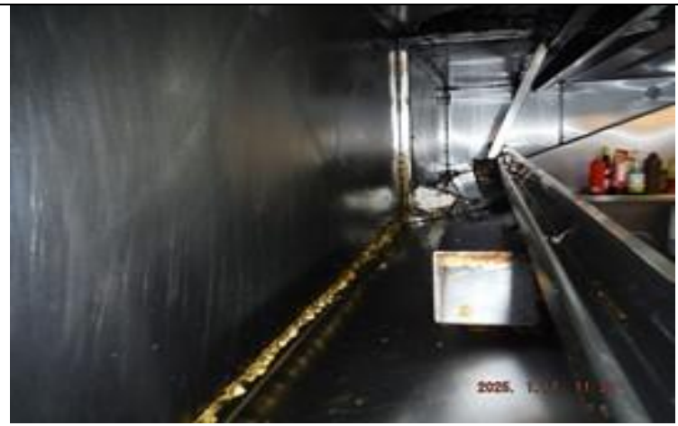
1. Canopy plenum (Main Extract) after
