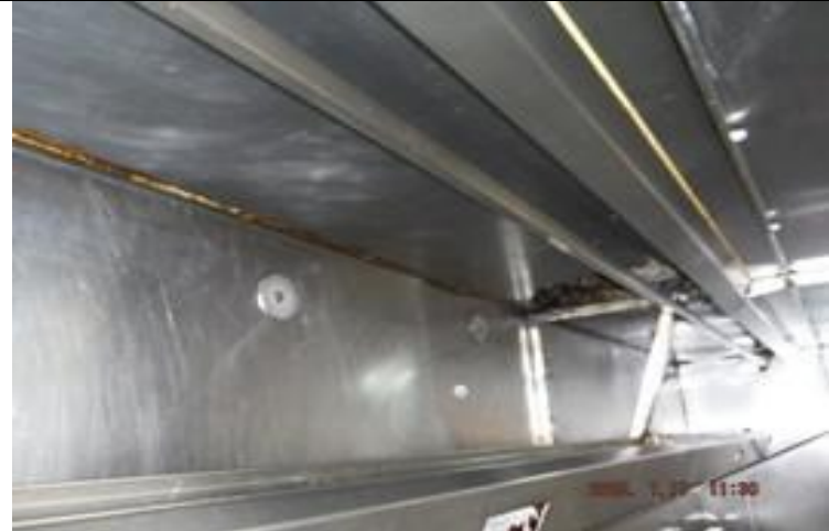
1 Canopy plenum (Main Extract) after
