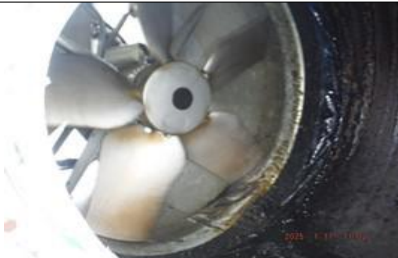
5. Duct upstream of fan before
