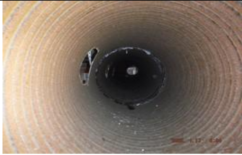
4. Ductwork Midway between canopy and fan before
