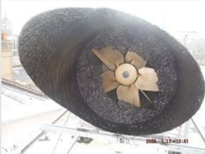
PICTURE SHOWS GRILLE SECTION REQUIRES REPLACING
