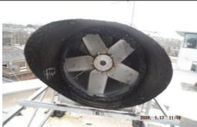
7 Duct downstream of fan after
