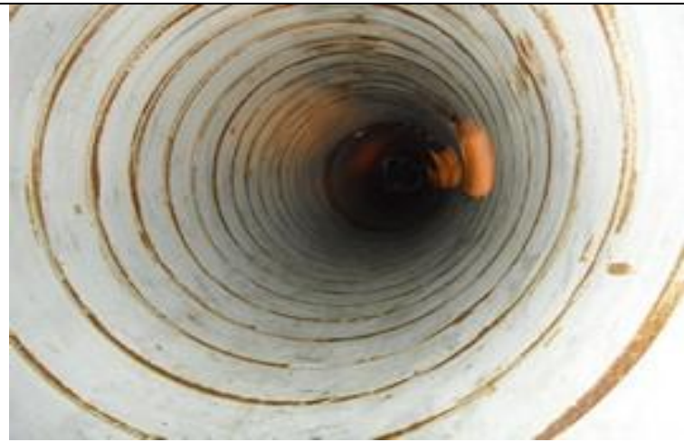
4. Ductwork Midway between canopy and fan after
