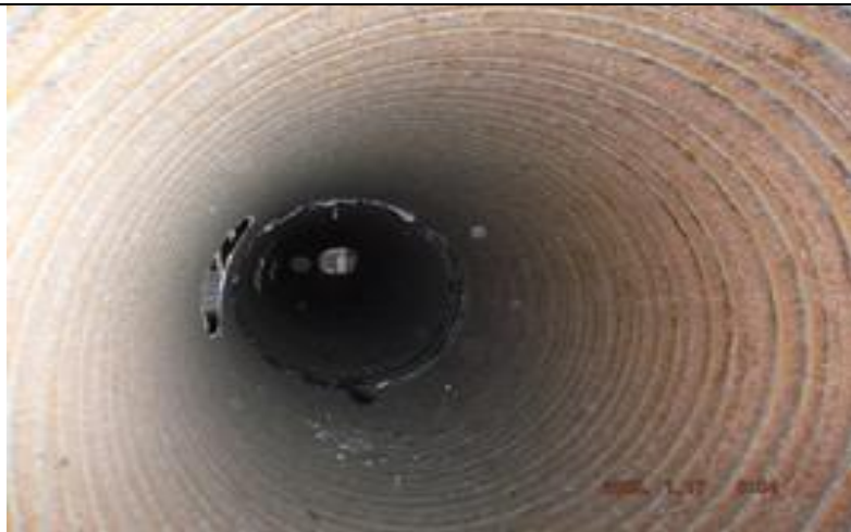
4. Ductwork Midway between canopy and fan before
