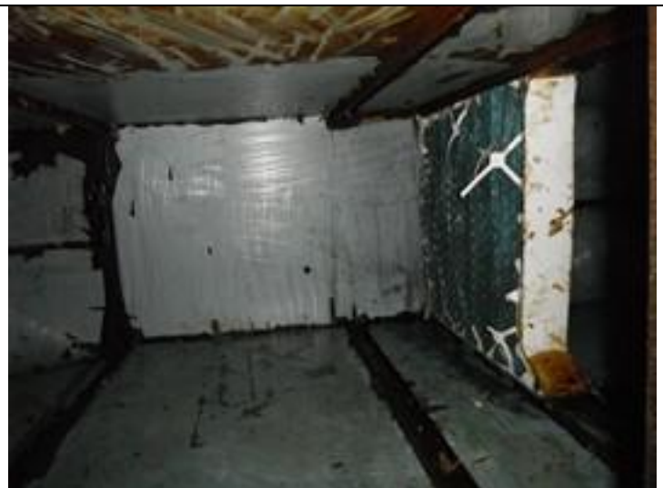
Filter box after
