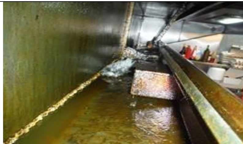
1. Canopy plenum (Main Extract)before
