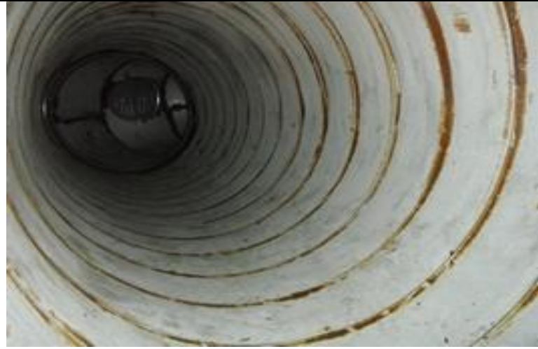
4. Ductwork Midway between canopy and fan after
