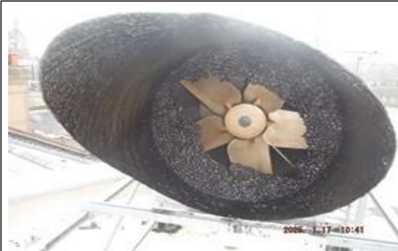
7 Duct downstream of fan before
