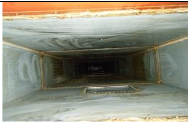
4.Ductwork Midway Between Canopy and Fan after
