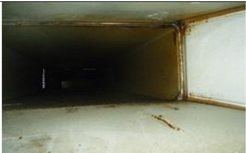
4. Ductwork Midway Between Canopy and fan before
