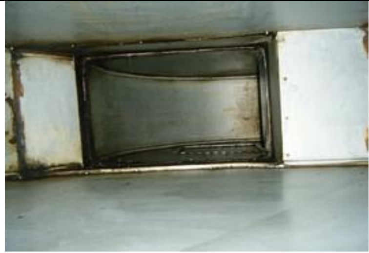
4. Ductwork Midway Between Canopy and fan after
