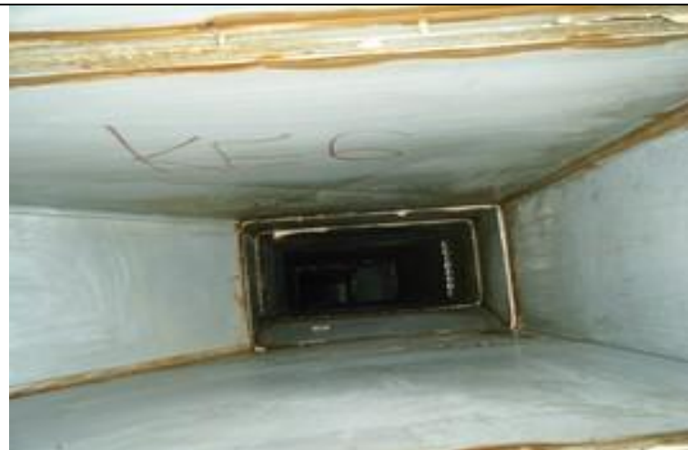
. 4. Ductwork Midway Between Canopy and fan after
