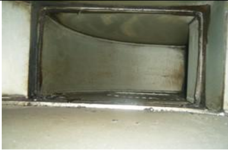
4. Ductwork Midway Between Canopy and fan before
