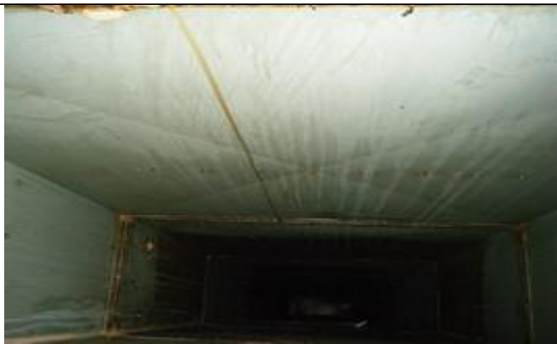
4. Ductwork Midway Between Canopy and Fan before
