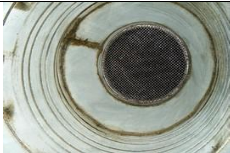
7. Ductwork Downstream of Fan after
